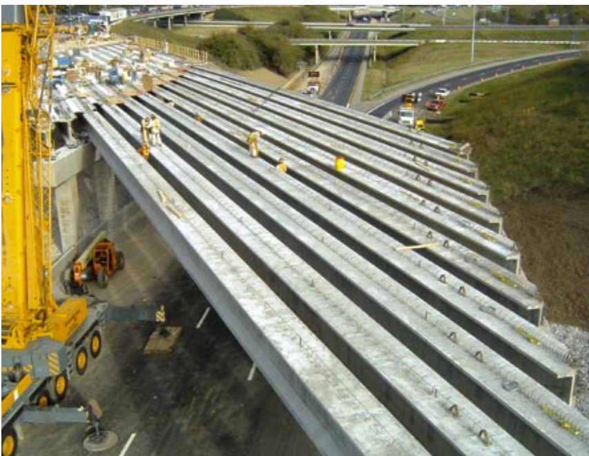
The intersection at which fire destroyed the bridge is perhaps the busiest in Alabama, carrying more than 100,000 cars daily.
